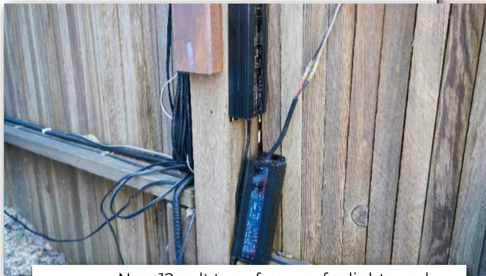
New 12-volt transformers for lights and sounds.
